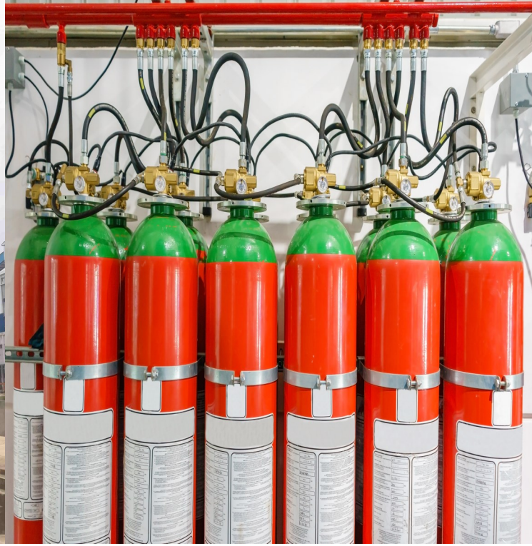
GAS SUPPRESSION SYSTEM
