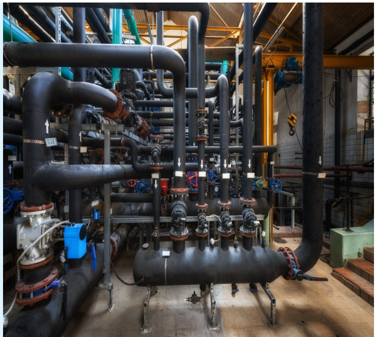
MECHANICAL UTILITY PIPING
