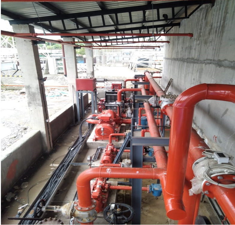
FIRE PUMP ROOM
