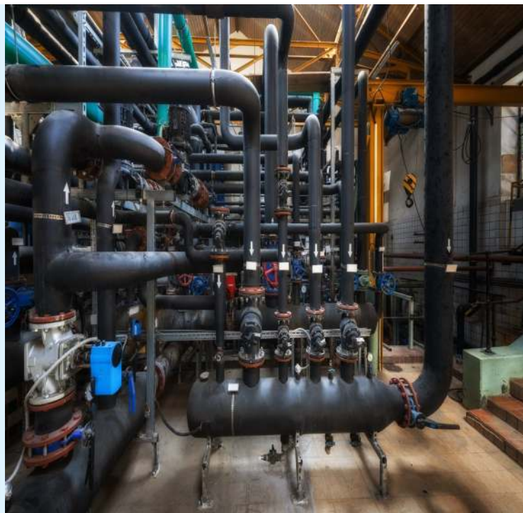
MECHANICAL UTILITY PIPING
