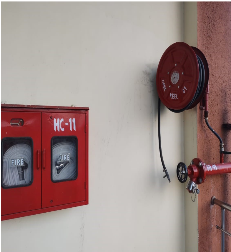
FIRE HYDRANT SYSTEM
