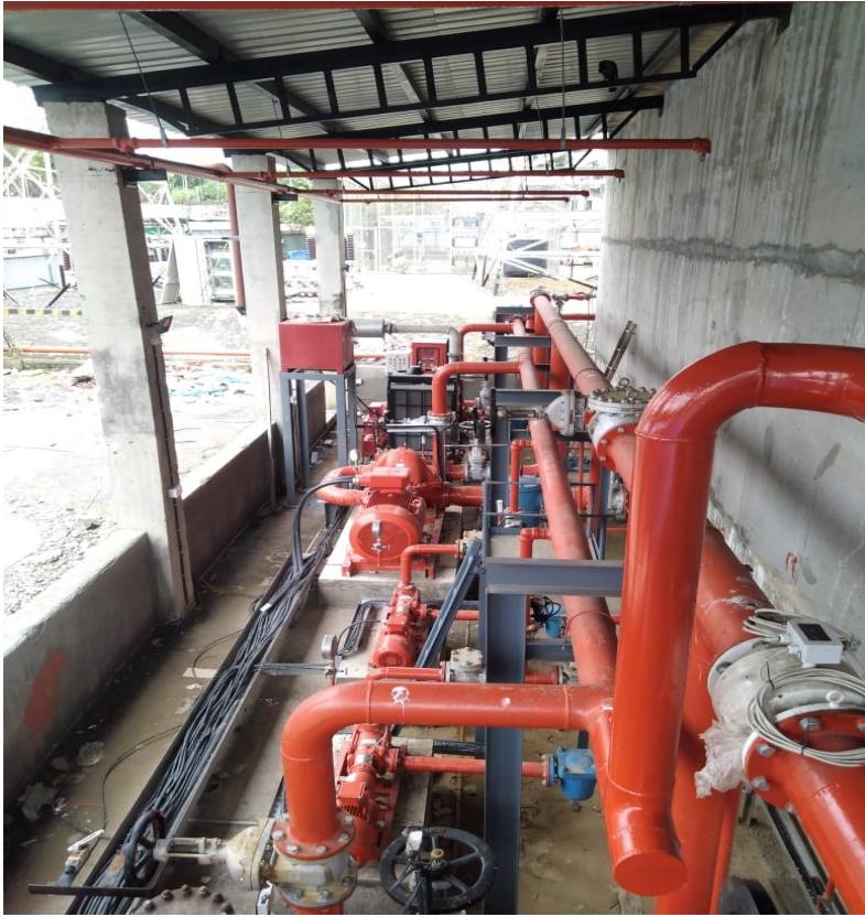
FIRE PUMP ROOM
