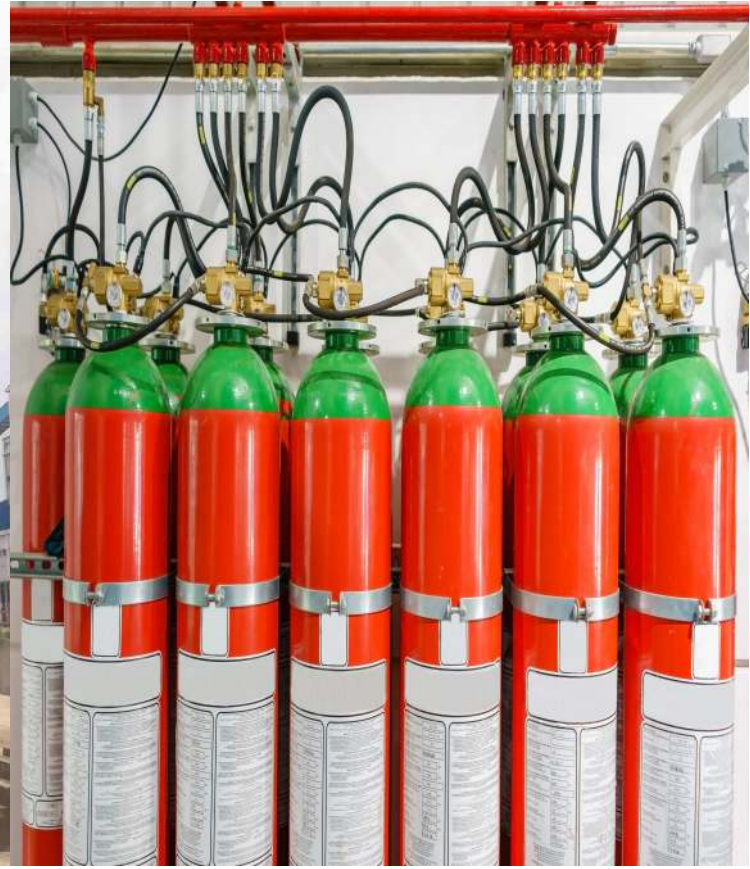
GAS SUPPRESSION SYSTEM
